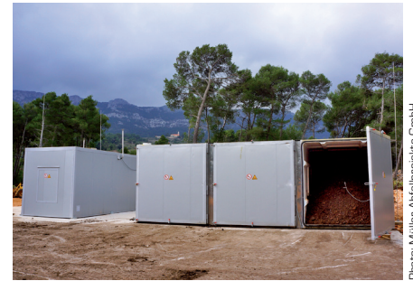
“Mobigas” container, biogas system for organic waste
