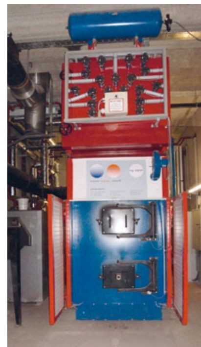
Biomass boiler of the project "Stift Kremsmünster" of Ing. Aigner GmbH Picture: Ing. Aigner GmbH
